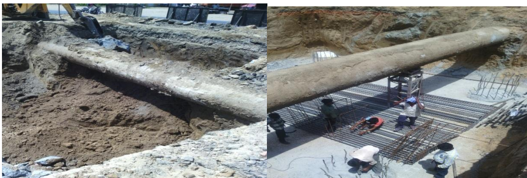
Figure: 1 Problem of Water Pipe Line below the Ground
