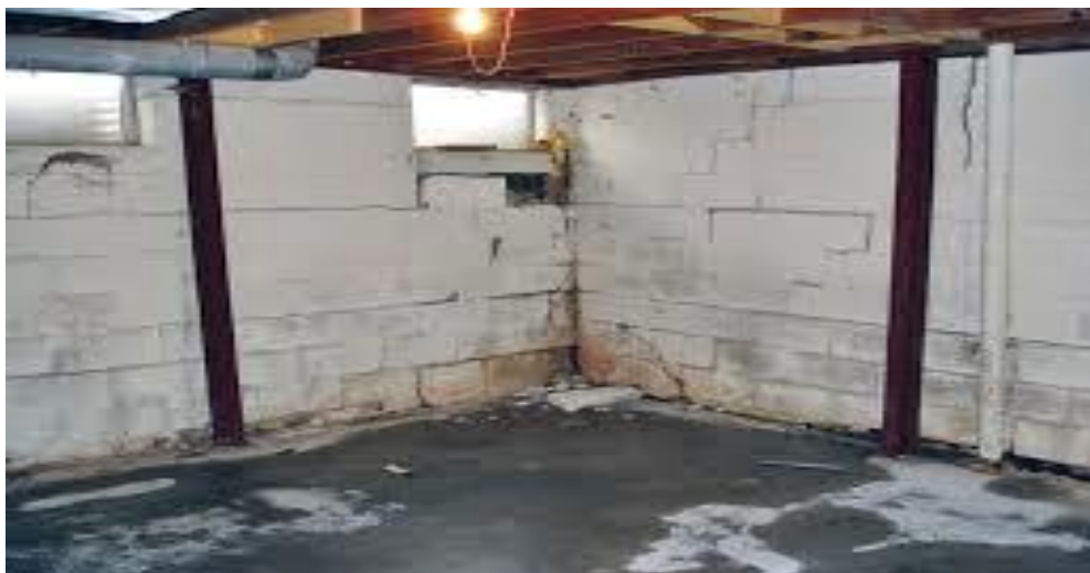
Figure 2. Deformation of basement flooring at nearby site
