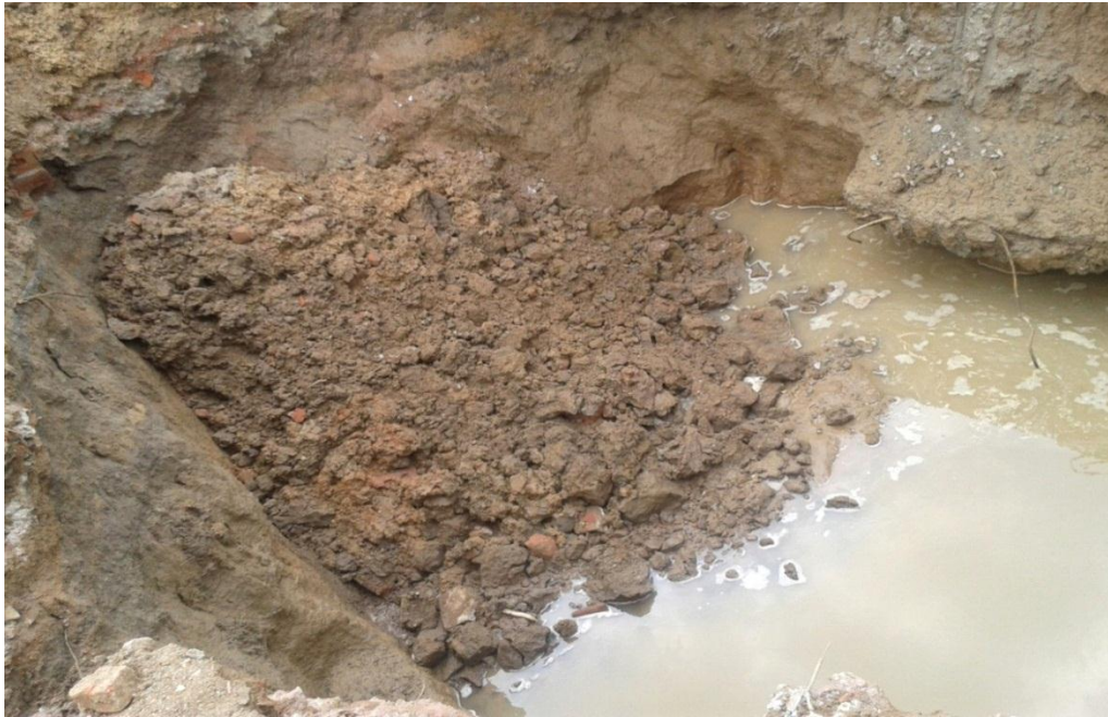
Figure 3 Failure of slump due to seepage water at ‘Silver Screen Multiplex’
